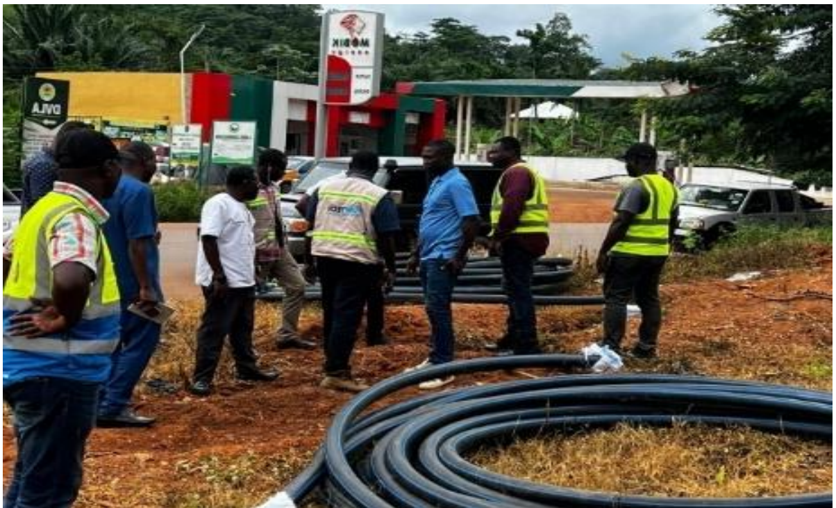
PUMPTECH Limited has installed a control valve.
