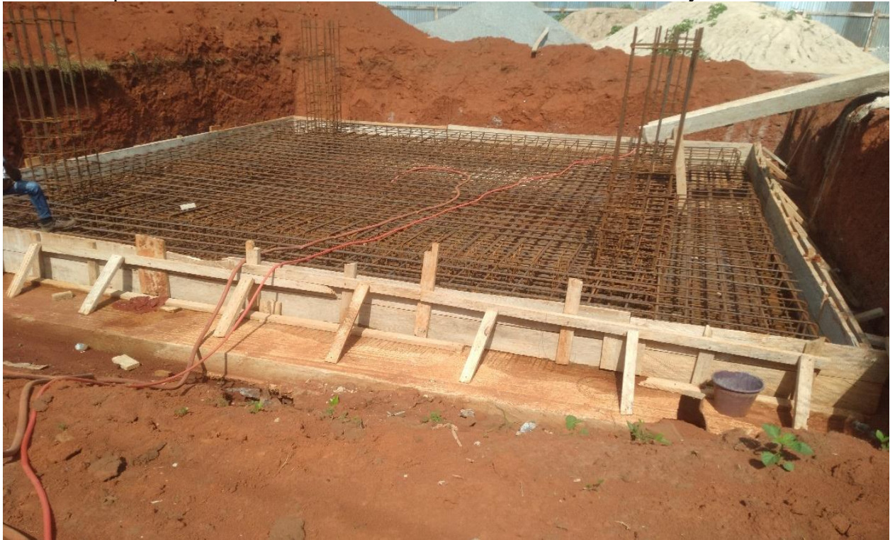
Formwork and foundation footing of 1no. High-Level Tank by BEDA Construction Engineers Limited
