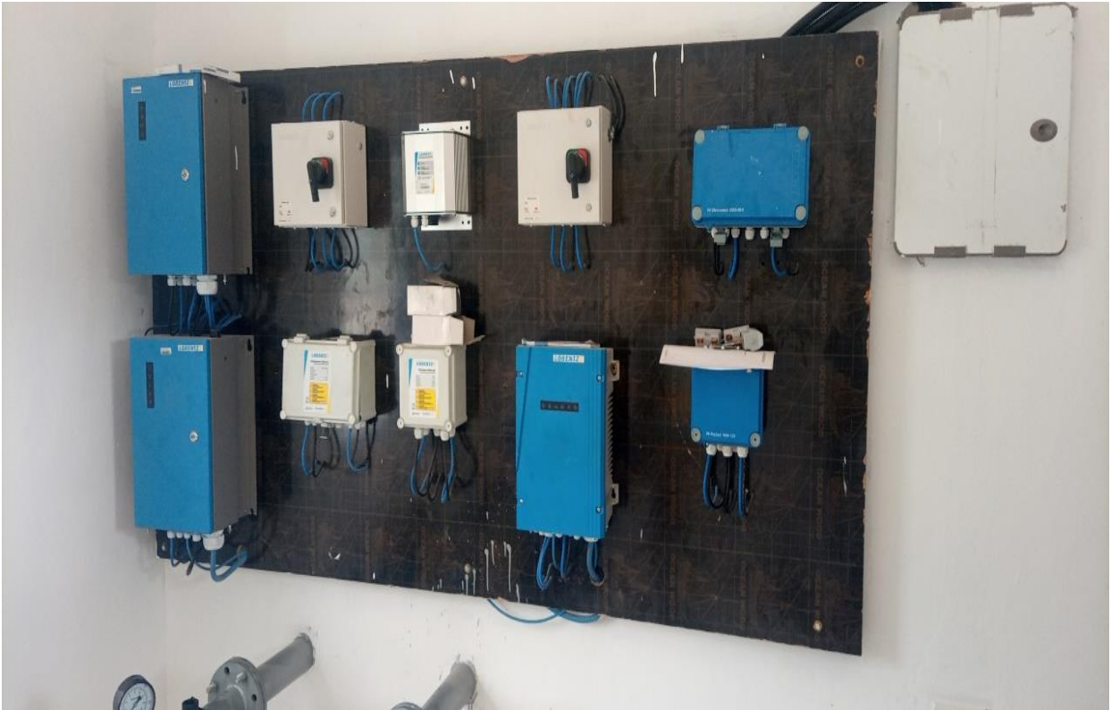
Installed Solar Farm and Pump Control Panels in Wulensi Water System by CAKSUNITY Services Limited
