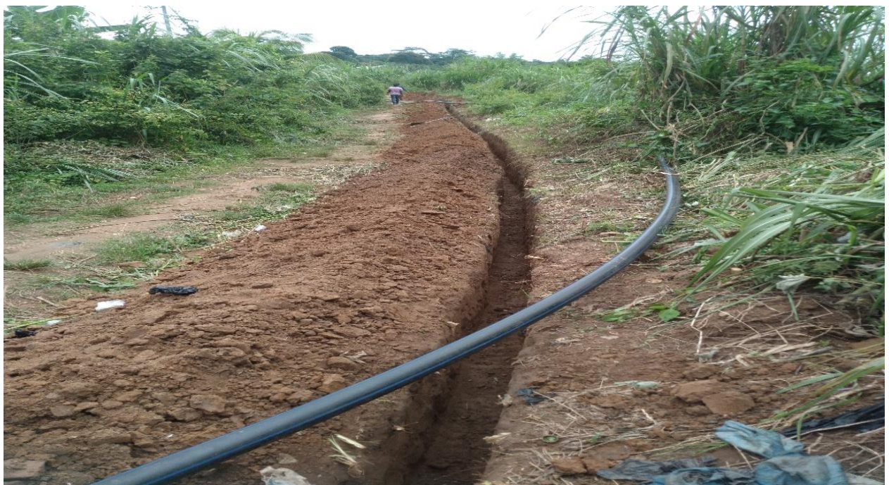
Laying of 2,000m long HDPE pipes to unserved areas in Hwidiem community by CWSA
